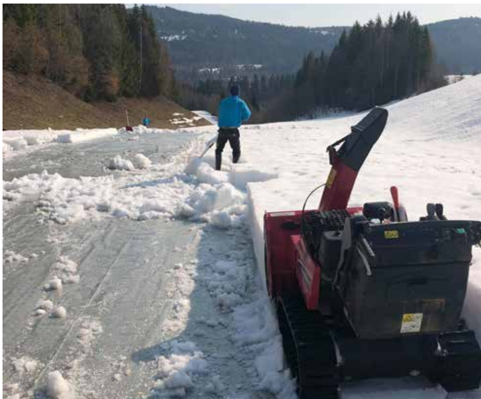
Photo 9. Snow removal above the impermeable cover may be necessary if O 2 concentrations are less than 2%. Photo: Mads Thers
